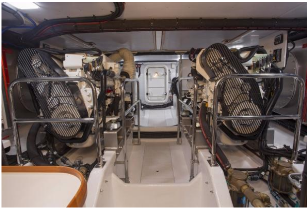
Engine room looking aft
