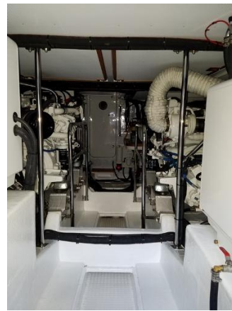
Engine room looking forward
