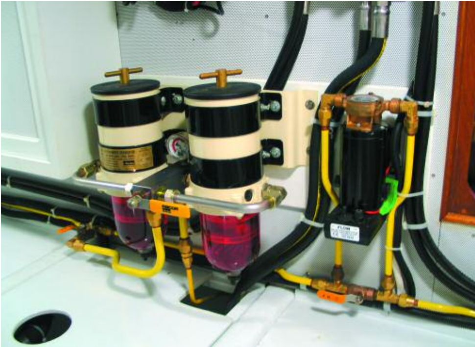
Main fuel filters and valves just inside the engine-room access hatch are within easy reach.
